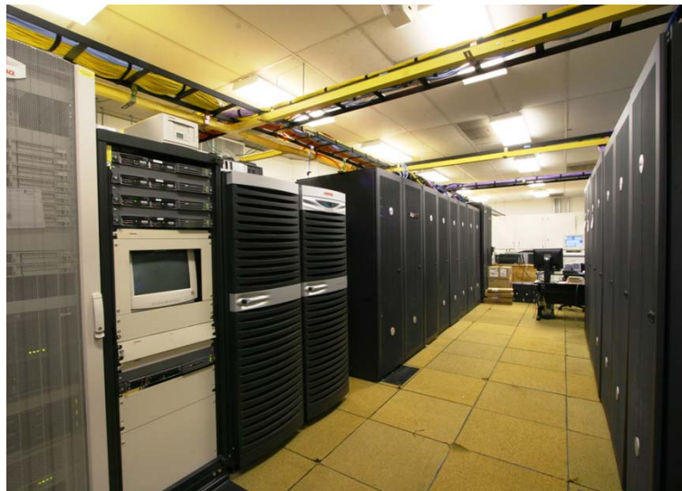
The EBRPSS network has 89 locations, 350 servers and 25,000 PCs
